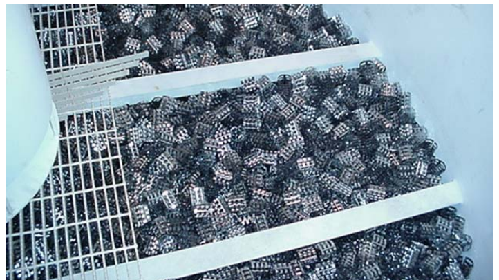
Fig. 6. A high surface to volume ratio packing without large contiguous surface area is installed in a 10 ft. diameter compact flotation vessel. Packing has been in service for over two years without plugging.
